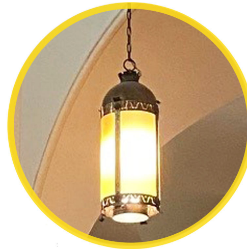
Type L Existing Surface mounted decorative lantern (glow + downlight)
